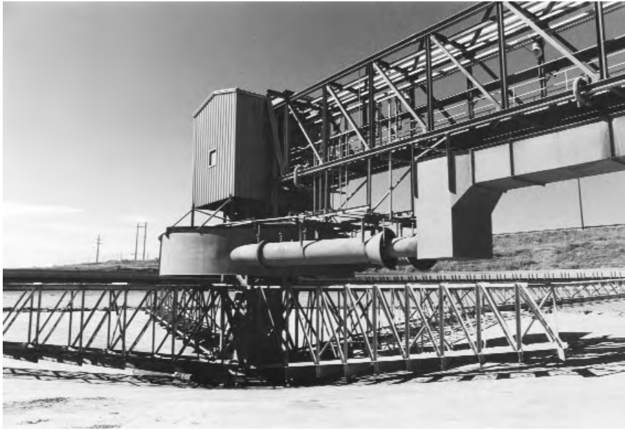
FIG. 18-92 E-Duc® Feed dilution system installed on 122-m-diameter thickener. (EIMCO Process Equipment Co.)
