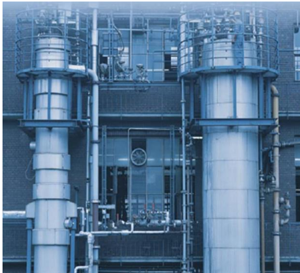
Figure 5.8 Two-step LOPROX plant for the pretreatment of 20 m 3 /h of effluent from the production of dyestuff at Bayer's Leverkusen factory.
